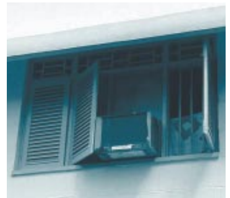
Aircons installed in bungalows and other private housing may be excluded.
